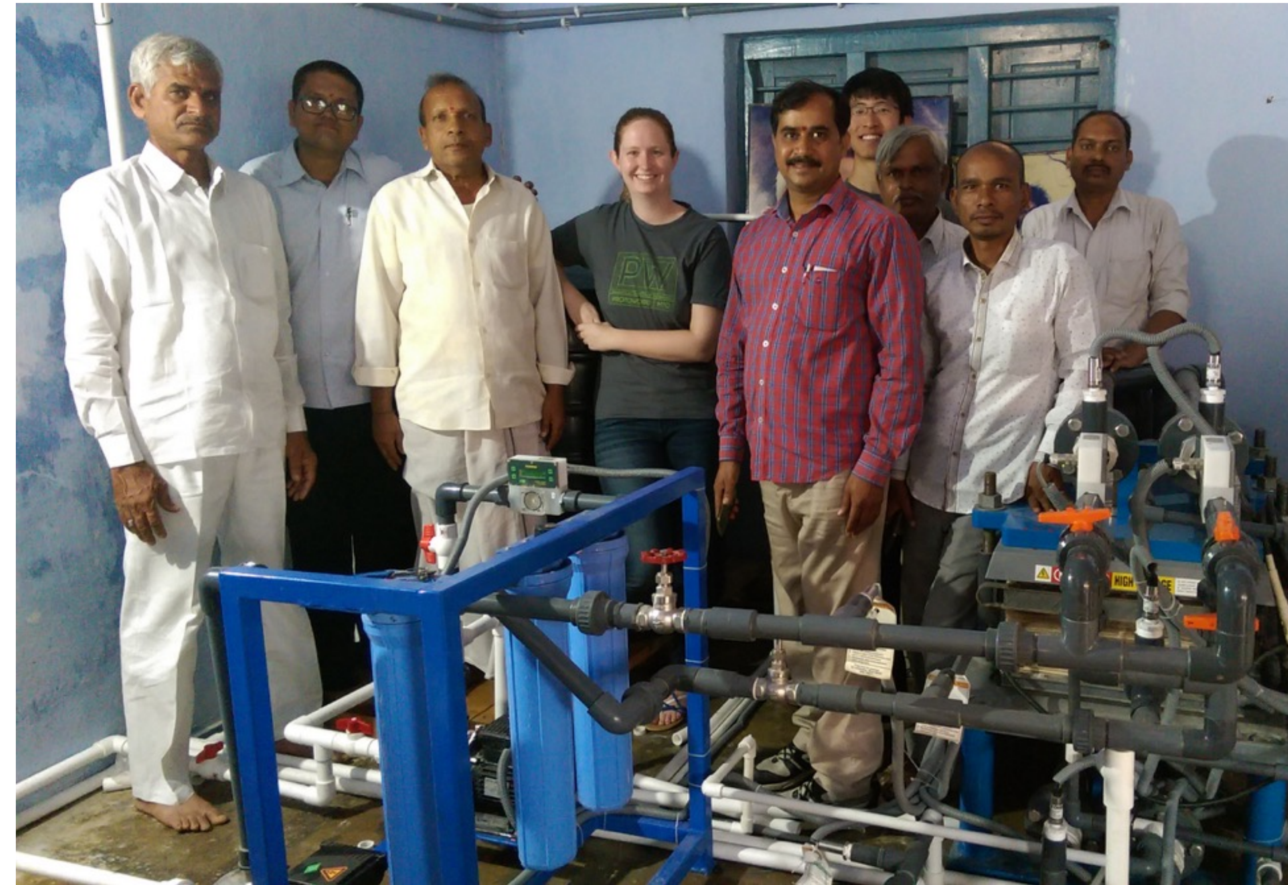
Optimized PV-EDR system in Chelluru, India
